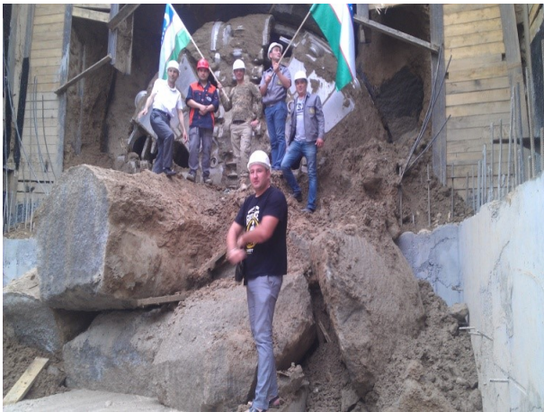
Fig. 5: Successful exit of the TBM into the dismantling chamber. When the tunneling is completed, surveyors and builders
